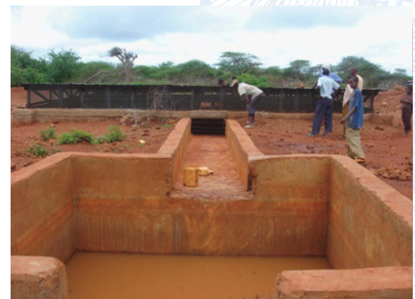
Completed water tank
