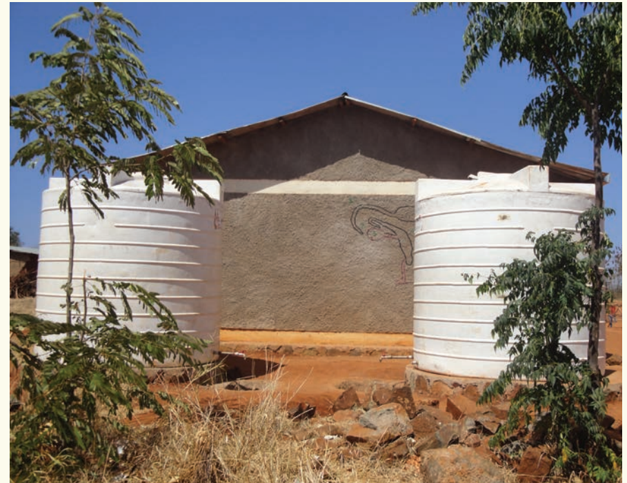
Two of the 24 storage tanks installed by IIRR in southern Ethiopia.
